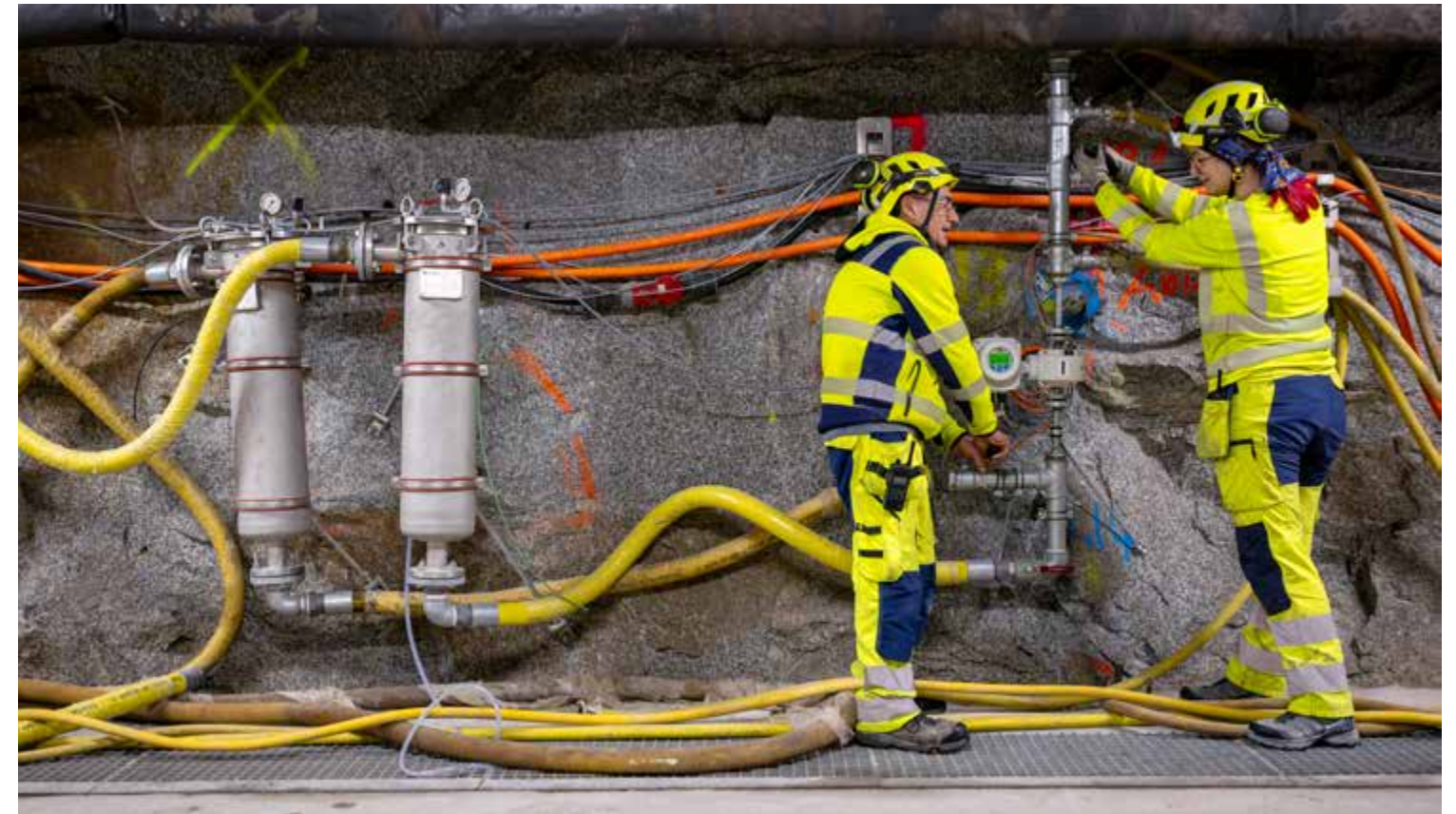
The BedrettoLab is full of pumps, sensors, cables and tubing for the many and various experiments conducted below the ground.
