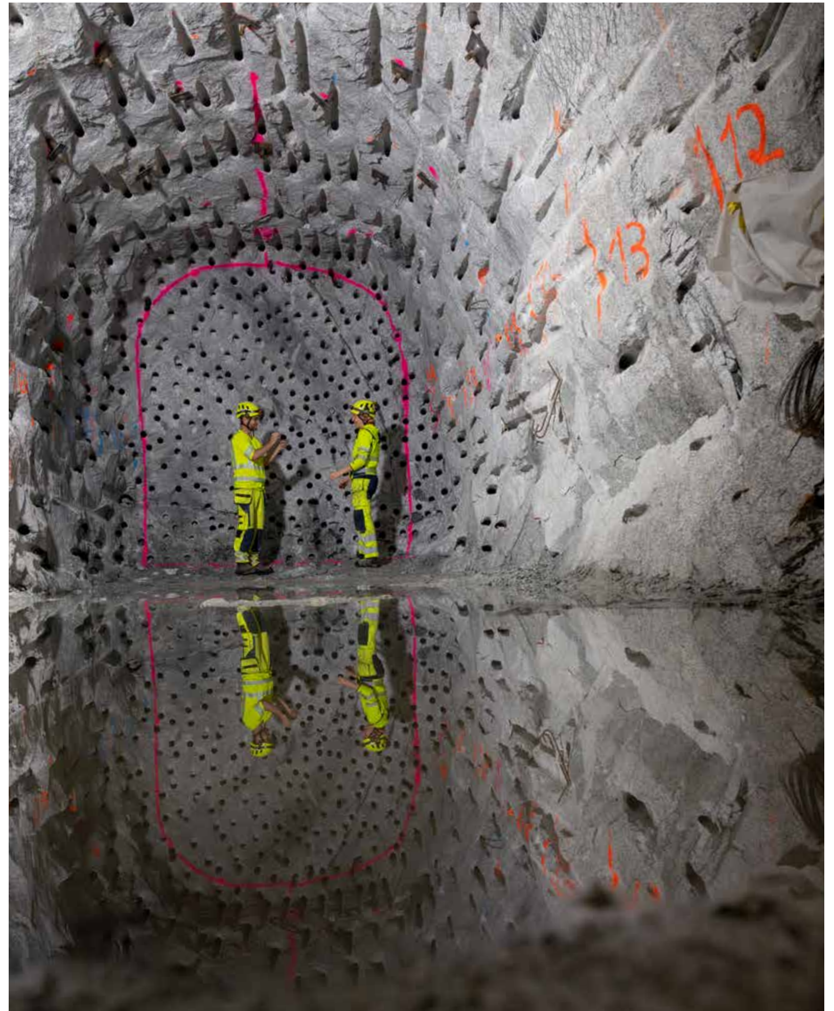
A new tunnel is under construction in the ETH Zurich's BedrettoLab in Ticino, offering even better conditions for earthquake research.
